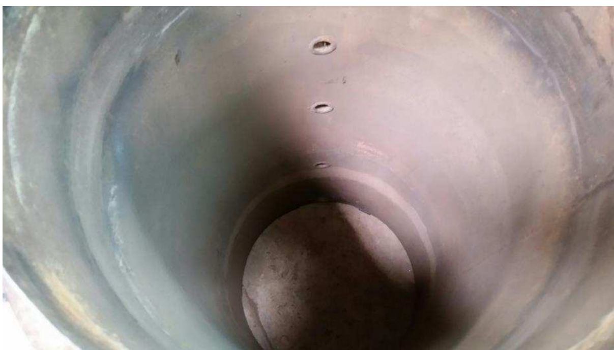
Figura 9 – Interior do Reator UASB
