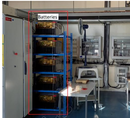
Figure 3-2: View of one of the battery banks (Zebra batteries) inside the powerhouse
