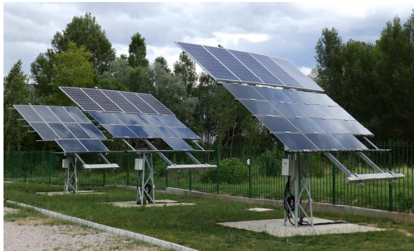
Figure 2-23: Different PV technologies installed on two-axis trackers.
