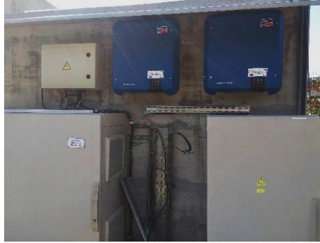
Figure 3-12: Inverters and instrumentation panels
