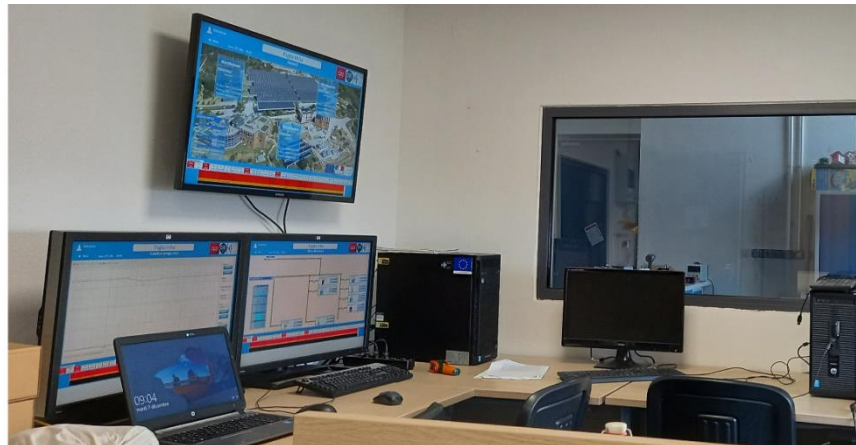
Figure 3-5: The control room inside the powerhouse
