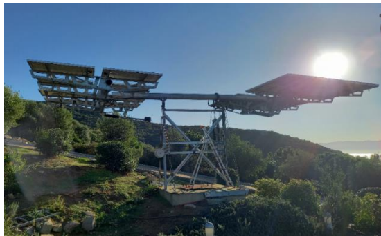
Figure 3-7: The PV tracker in its “rest” position
